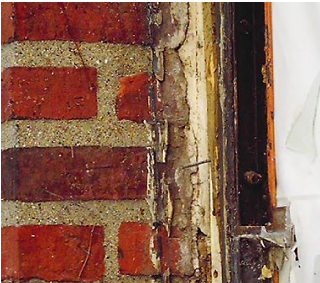
Example of decaying caulk and paint with evidence of PCBs.
